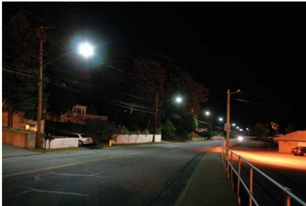
Induction lamps replaced high-pressure sodium lighting on Meridian Street in Groton, Conn. A remaining HPS lamp lights the parking area on the right in this photo.
